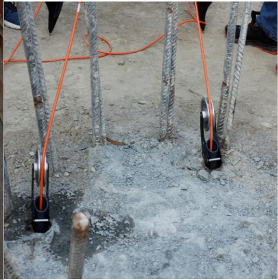
Probes under water filled tubes, total depth of one tube is 31m.
